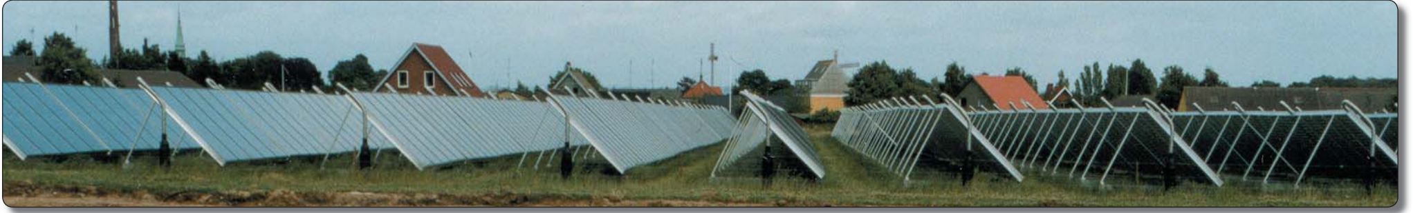
29% of the hot water in Marstal, Denmark is supplied by 18,365m 2 of solar-thermal collectors. Photo: Ide Seidelin, Ærø
