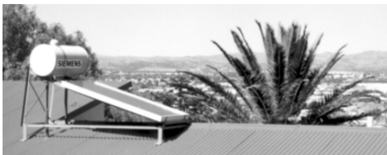
Almost 500 solar collectors have been installed in Namibia with a help of a loan scheme
