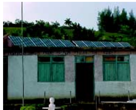
The photos show PV systems installed at different schools in Cuba.
