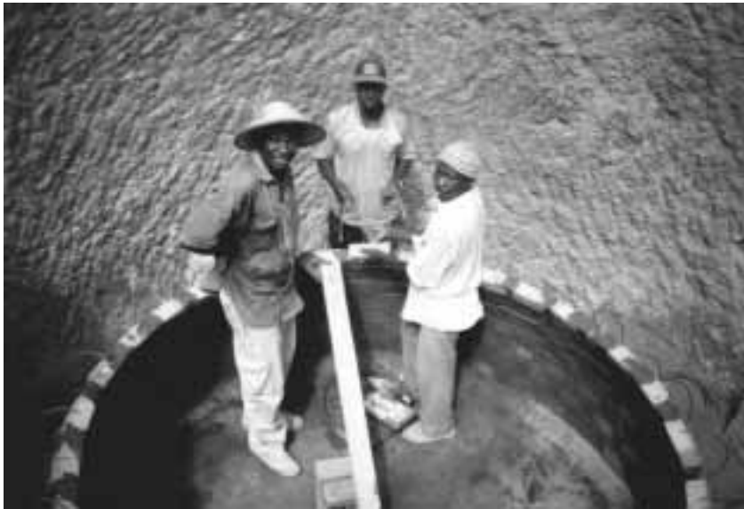
Training a local mason to build a biogas digester dome using locally made bricks.
