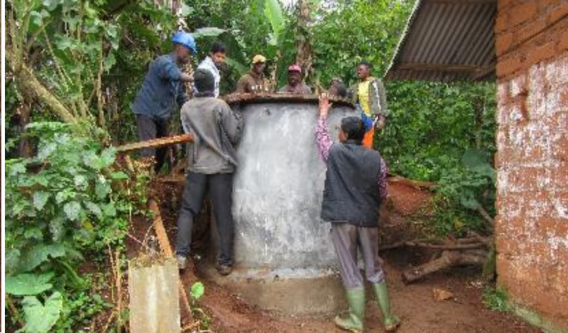
Rooftop Rainwater Harvesting
