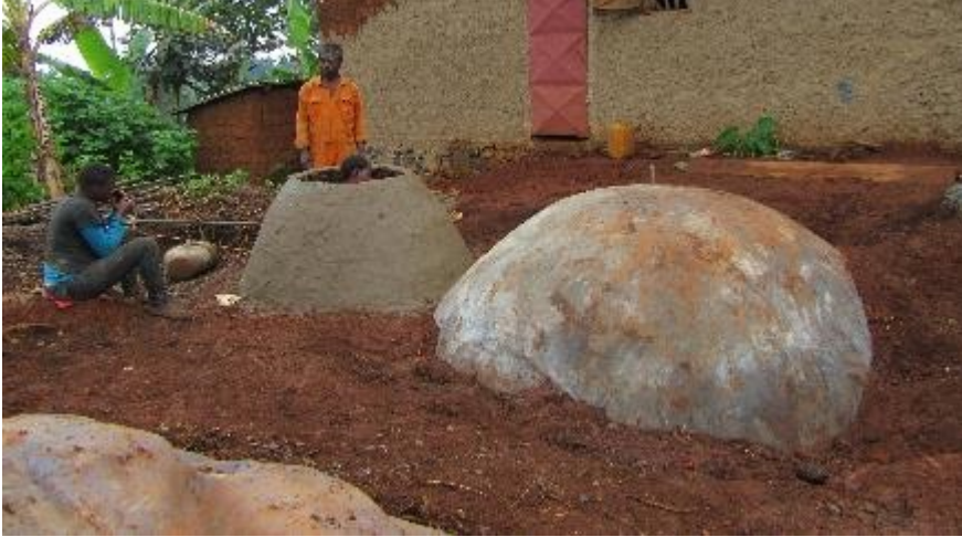
Bamboo reinforced cement Biogas Plant
