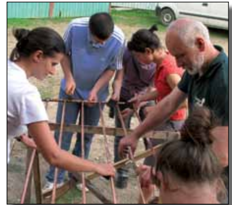
The Do-It-Yourself (DIY) solar collectors built by Ion Zamfir (right) and a team of trainees. All six solar collectors on the roof of the centre were made by teams of trainees who came to learn about renewable energy in our beautiful environment. The collectors are effective and cheap to produce using just a few tools, some materials available in all plumbers' shops with a little bit of technical skill.
