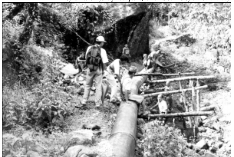
Local people are participating to lay down the headrace pipe of a micro-hydro power plant, which is owned by the community.
