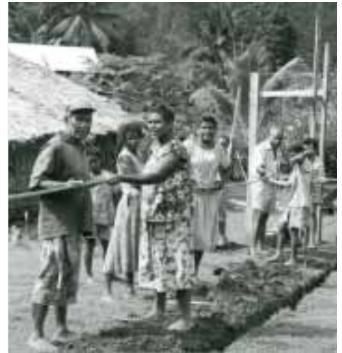
Wiring micro-hydro, Solomon Islands. Photo: Robert Wadell, APACE.
