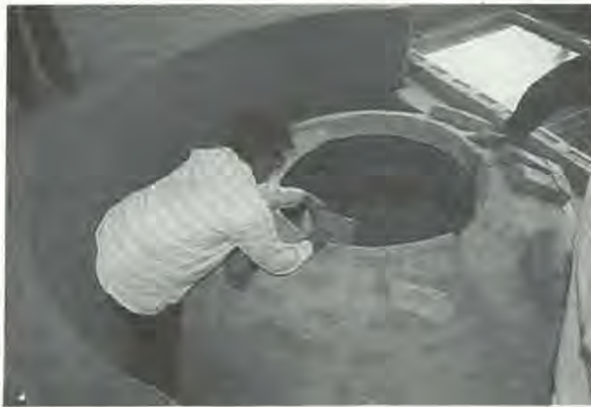
Cement and bricks with plaster inside. Bricks can be replaced with weaved bamboo and cement.
