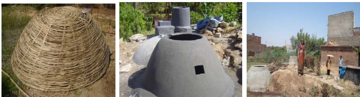
Pictures: Bamboo basket as reinforcement for cement dome for biogas, biogas plants under construction, finished biogas plant covered with soil
