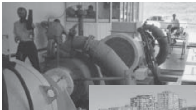
A small 800-kW grid-connected hydro power plant installed in 2000 in Armenia.
