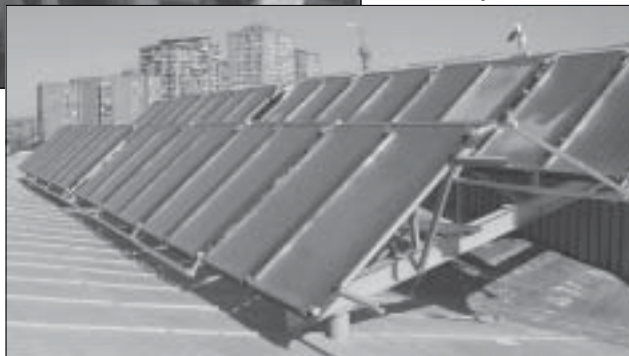
The largest solar water heating system in Armenia with total area of 64 m 2 , manufactured and installed in 2002 by SolarEn LLC.
