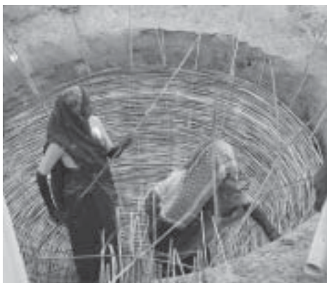
Photo (Right-top): Construction of Deenbandhu biogas plant with a dome made of bricks, in India a job for men, but the produced biogas benefits women who are cooking.
