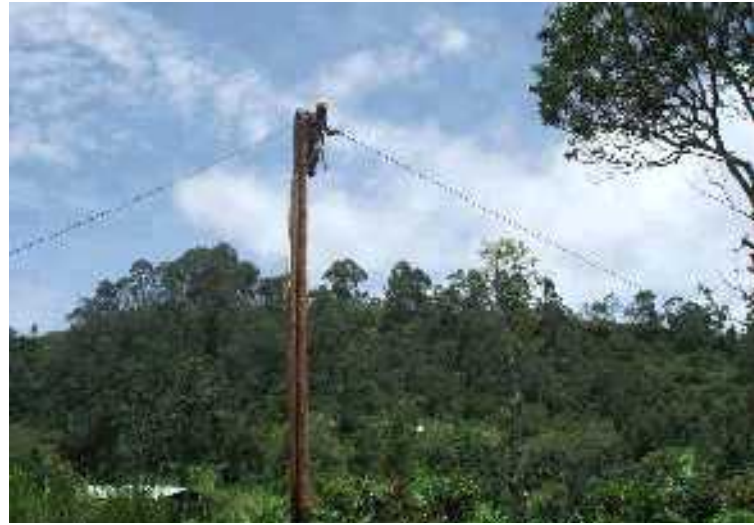
Connection of the grid in Tchouandeng
