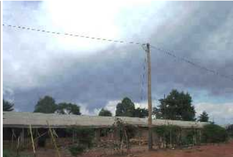
A primary school electrified with ADEID'MHP
