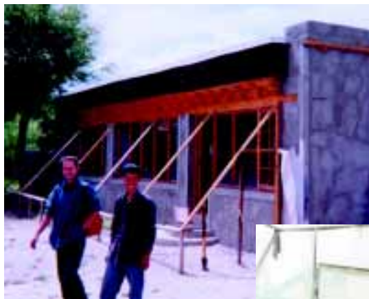
Construction of a solar extension at the Pashmina wool processing centre. A bioclimatic building for better conditions of work.
