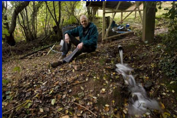
Llangynidr Hydro (installed Oct 2007)
