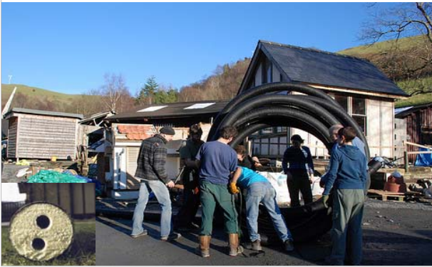
UK's first fully renewable district heat main
