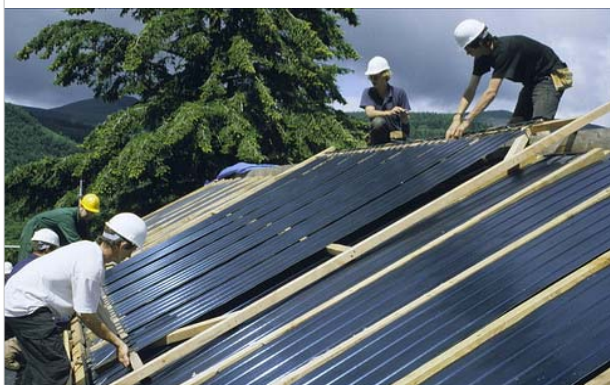
UK's largest solar thermal roof
