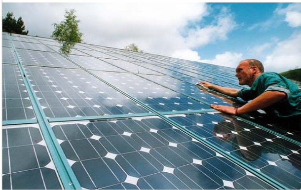
UK's first building Integrated PV roof
